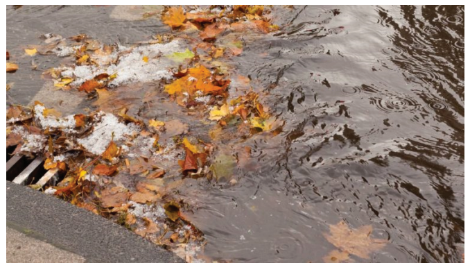
Blocked drains cause flooding.
