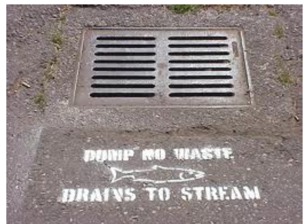
Clean and marked storm drain
